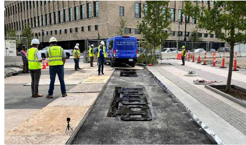
15 th St. Static Charging Installation
